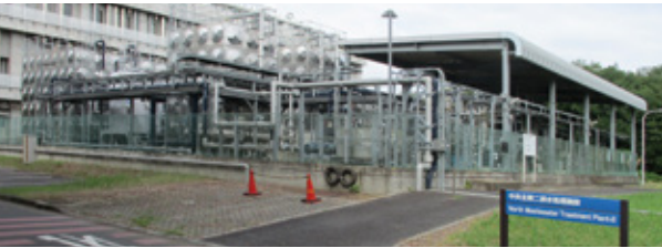
Wastewater treatment facility in AIST Tsukuba
