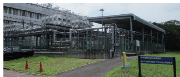
Wastewater treatment facility in AIST Tsukuba
