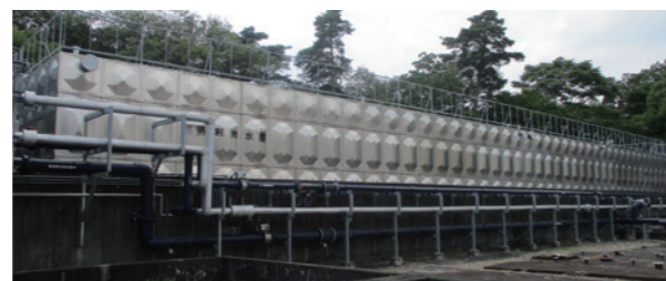
Recycled water tank in AIST Tsukuba
