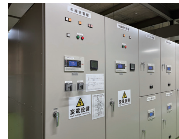
After substation facility renovation
