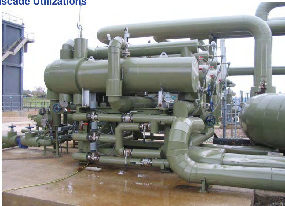
Main heater on secondary steam for Cheese factory
