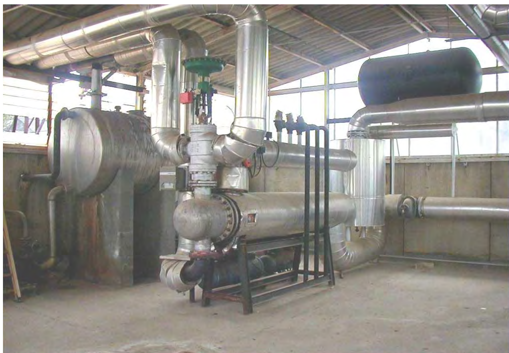
Green houses Heater
