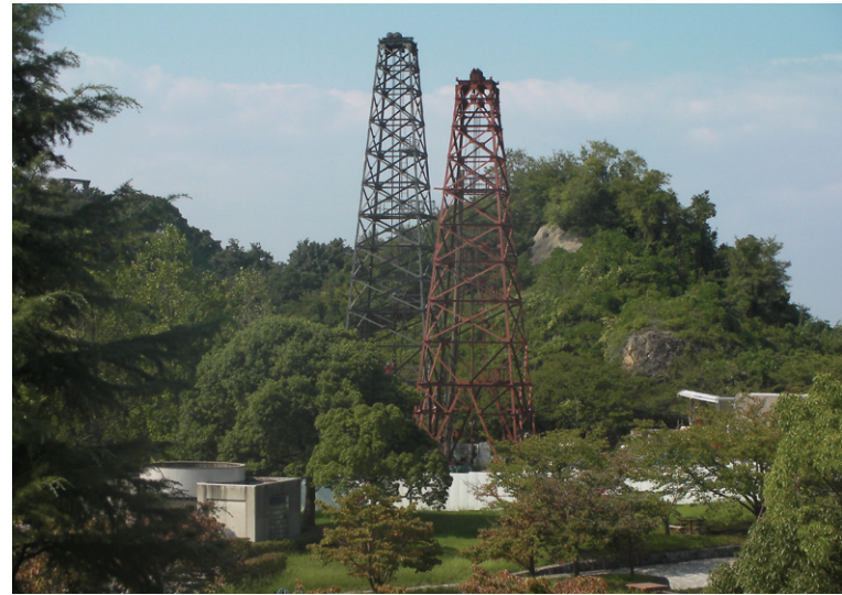
▲ AIST observation well (A photo during construction. Upon completion, the derrick will be dismantled)
