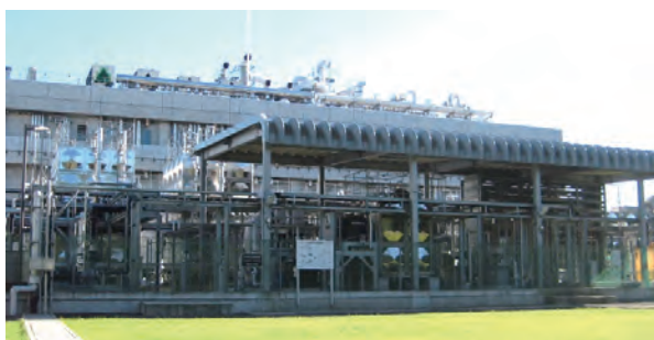
Wastewater treatment plant at AIST Tsukuba
