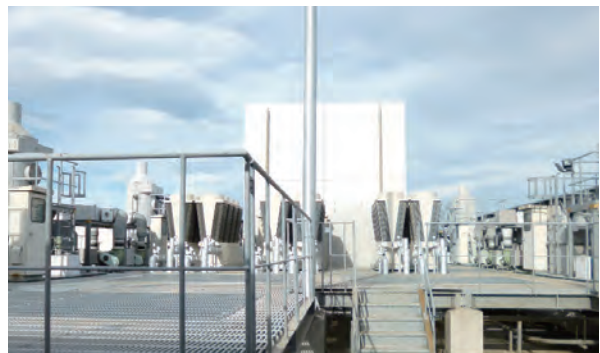
Tsukuba Central 3 heating equipment: Upgraded from gas-powered hot/cold water generators (top) to electric air-cooled modular chillers (bottom). The upgrade is expected to provide an energy saving of 54%.
