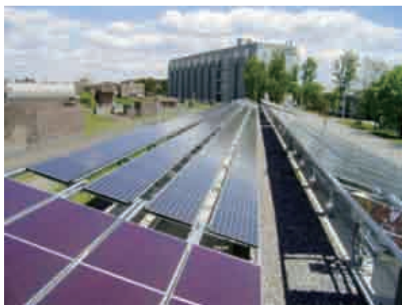
Mega solar town "Taiyo No Oka (Hill of the Sun)" at AIST Tsukuba
