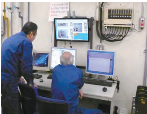
Fig. 2 PC control system installed in the control room
