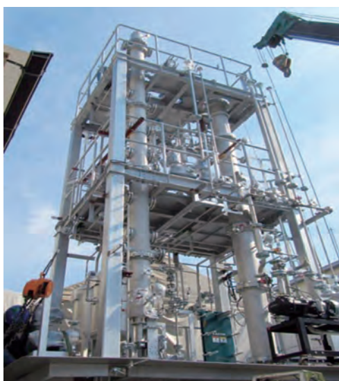
Fig. 17 Bench plant of CF-HIDiC under installation [10] mash column (right) and HIDiC main column (left)
