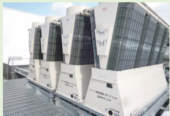
High-efficiency modular chiller system
