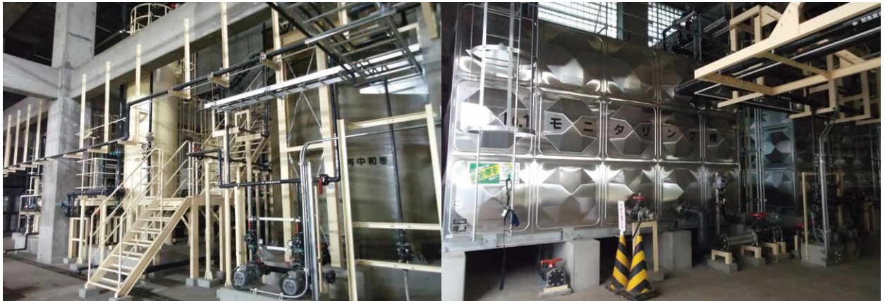
Wastewater treatment plant at AIST Tsukuba
