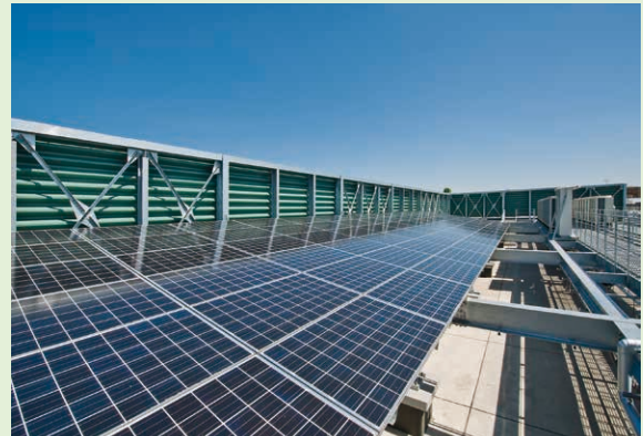
Solar power-generating panels installed on the roof of the research base building
