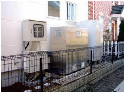
Fig. 3 The installed air-conditioning and hot water supply system. From left to right: measurement equipment, heat pump and hot water tank.
