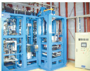
Fig. 1 : Experimental apparatus for supercritical CO 2 cleaning
